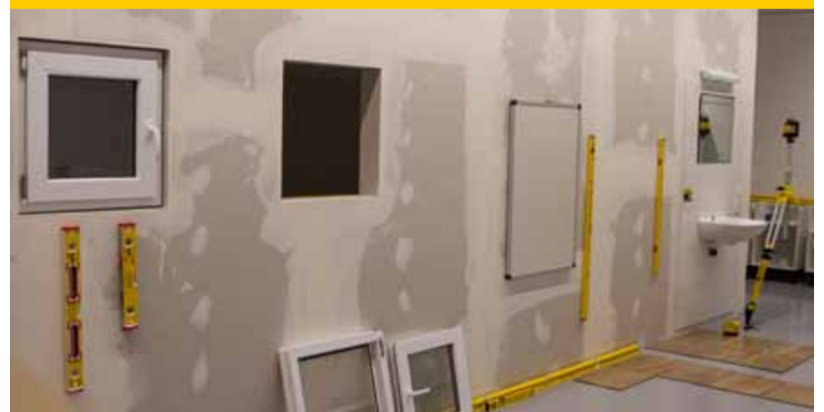
Various interior construction jobs, such as installing windows, laying tiles, electrical and plumbing installations, are demonstrated on the drywall.
